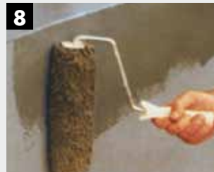
8 Apply two protective coats of KEIM Concretal-C. Two undiluted coats applied by brush, roller or airless sprayer.
