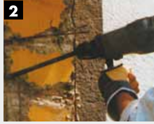
2 Exposing corroded steel reinforcement
