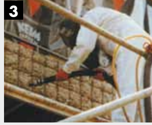
3 Cleaning the steel reinforcement by dry blasting with solid blasting media. Degree of rust removal, Sa 2½ to DIN EN 12944-4
