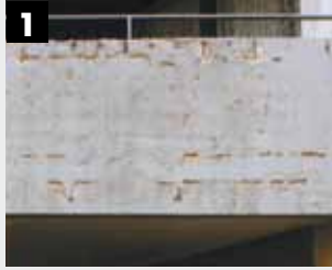
1 Typical decay of inadequately protected concrete
