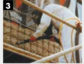
3 Cleaning the steel reinforcement by dry blasting with solid blasting media. Degree of rust removal, Sa 2½ to DIN EN 12944-4
