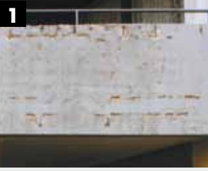
1 Typical decay of inadequately protected concrete
