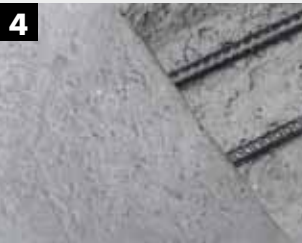
4 Fill defects with mineral KEIM Concretal-Universalmörtel in the prewetted substrate, use without specific corrosion protection and bonding bridge. Layer thicknesses of 0.5–5 cm are possible, multiple layers must be used from a thickness of approx. 2.5 cm. KEIM Concretal-Universalmörtel-S can be directly smoothed.
