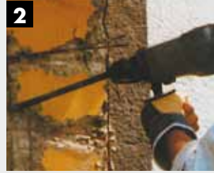
2 Exposing corroded steel reinforcement
